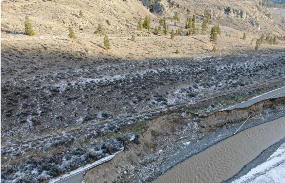
FIGURE 4: DAMAGE TO HIGHWAY 8 AT SITE 9 (Photo taken on December 12, 2021)
