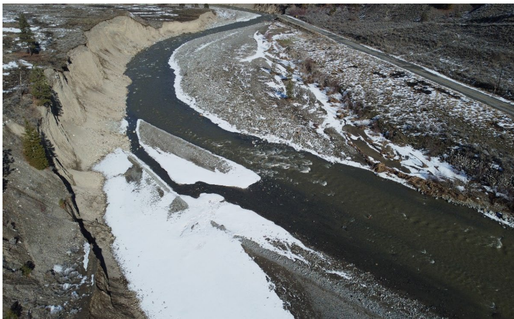
FIGURE 10: DAMAGE TO NVR (USED AS TEMPORARY HIGHWAY 8 ALIGNMENT) AT SITE 10C (Photo taken February 15, 2022)
