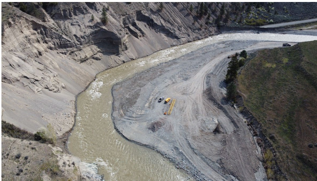
FIGURE 12: DAMAGE TO NVR (USED AS TEMPORARY HIGHWAY 8 ALIGNMENT) AT SITE 10D (Photo taken April 14, 2022)
